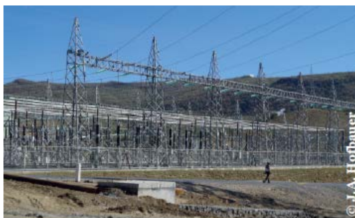
Olkaria geothermal plant, Kenya.
