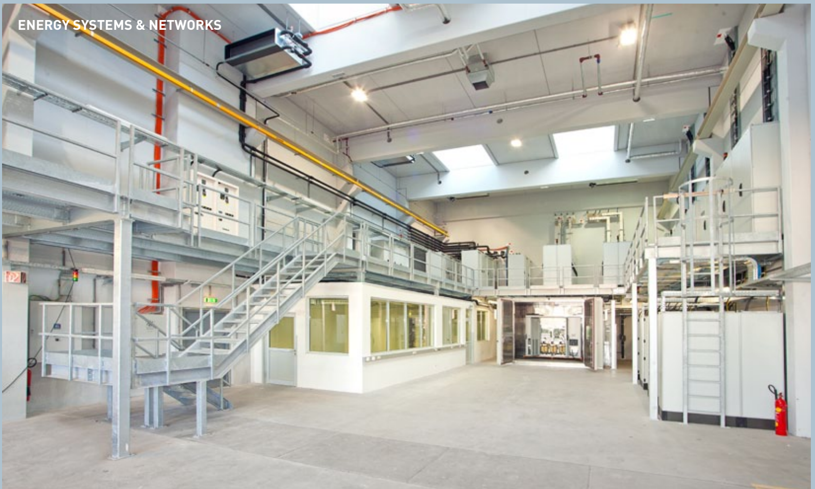
AIT SmartEST Laboratory Photo: AIT Austrian Institute of Technology GmbH/Harry Krischanz
