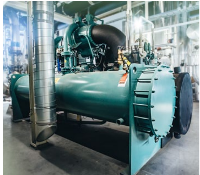
Refrigeration machine Photo: Infineon Technologies Austria
