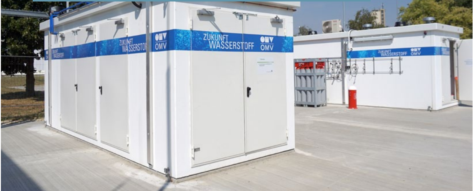
Wind2Hydrogen pilot facility at OMV site in Auersthal, Lower Austria Photo: OMV
