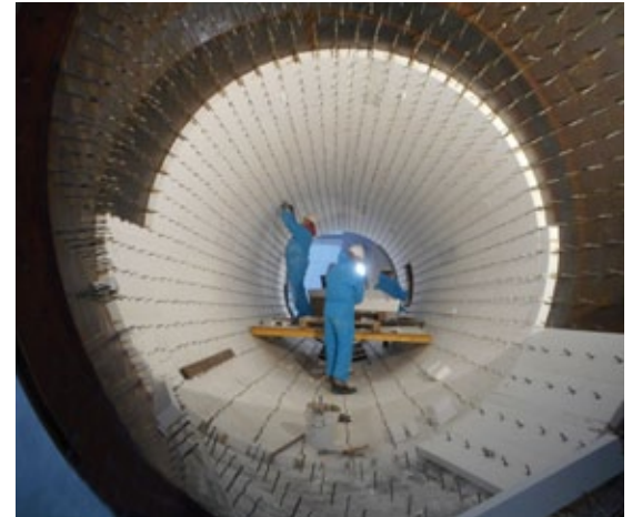
Fireproof refractory lining for the air discharge duct Photo: voestalpine Stahl GmbH
