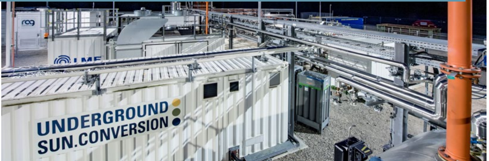
RAG's plant in Pilsbach/Upper Austria Photo: RAG Austria AG/Karin Lohberger Photography
