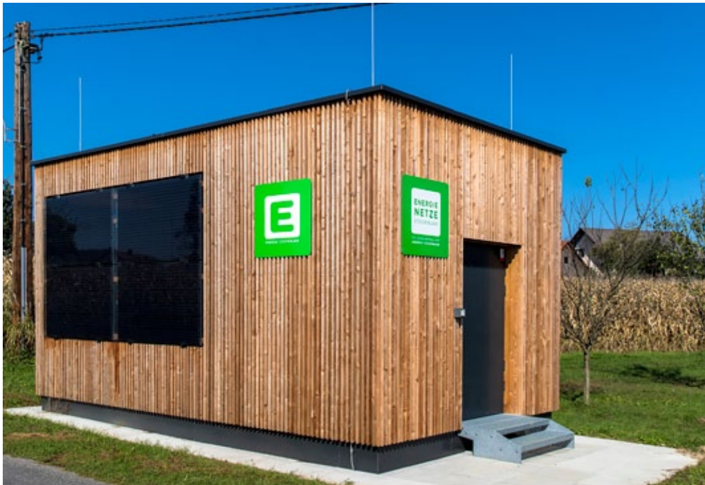
Central storage system Heimschuh Photo: Energie Steiermark/Symbol
