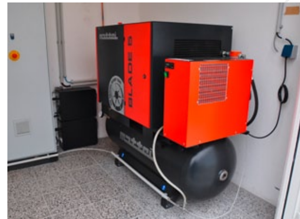
Wind2Hydrogen pilot facility Photo: OMV
