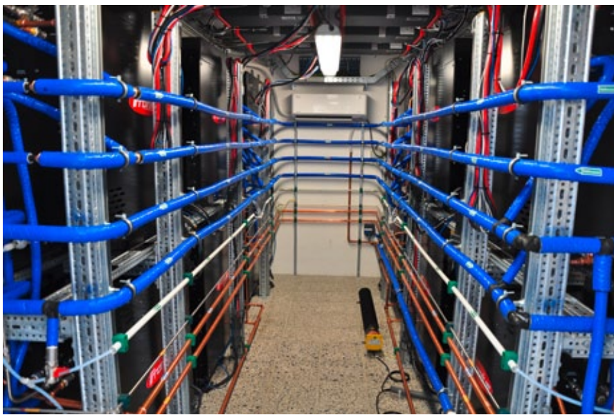
Wind2Hydrogen pilot facility Photo: OMV
