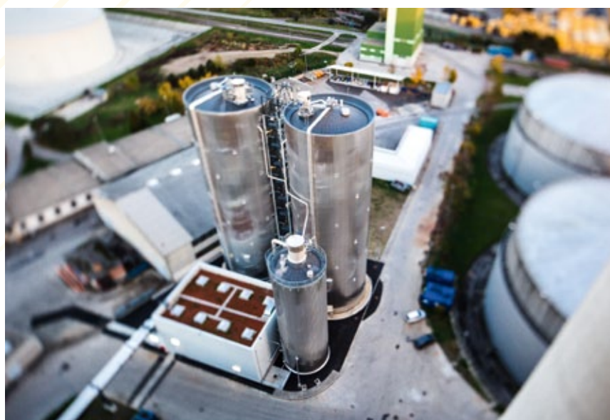
High pressure heat storage facility, Simmering power plant Photo: Wien Energie/Ian Ehm
