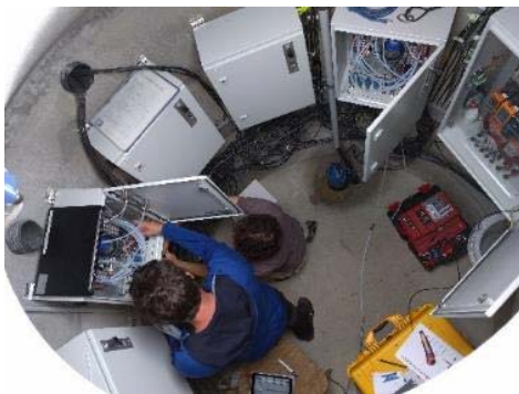
Figure 8 Belowground control-unit of the depth profile trace gas measurements
